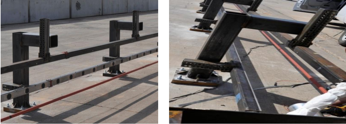
Figure 5. Instrumentation Rail Support Structure and Insulated Rope
